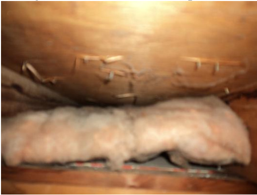
Photo #4a Add closed cell spray foam to the sloped ceiling when the roof is to be replaced
