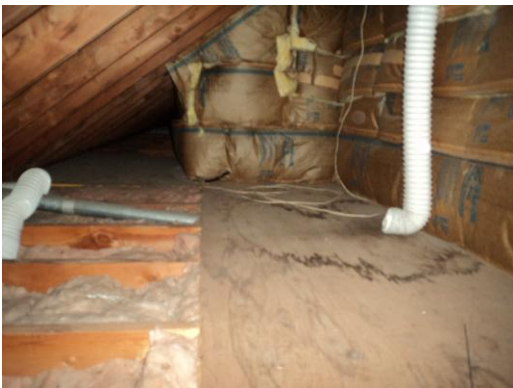
Photo # 2 Remove existing batt insulation and air seal with closed cell spray foam. Replace bath fan material with insulated type and vent to the outside
